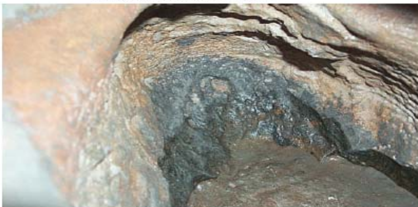
Close-Up View of Cavity
