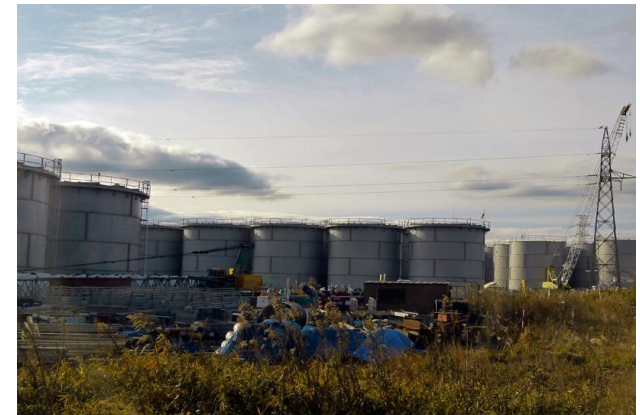
Storage tanks for contaminated water, a major challenge at the Fukushima Daiichi site. Source: IAEA
